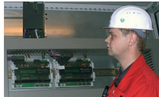
Helmut Blekker, project superintendent at ExxonMobil, takes a look at the control cabinet with the process automation station (top) and the Profibus/MP-Bus gateways (bottom).
