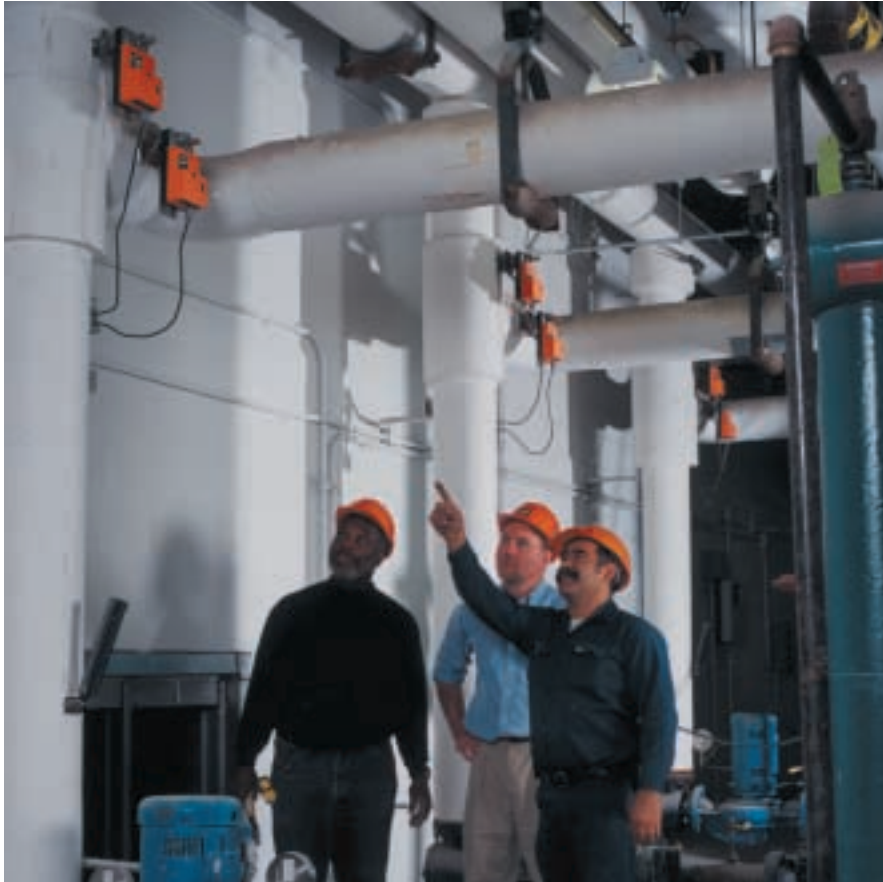
Steve Handleman, Belimo Sales Manager, inspects Belimo Butterfly Valve in boiler room of New York Post printing facility.
