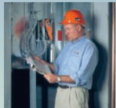
Steve Handleman, Belimo sales manager, inspects installation of AF Series Spring Return Air Damper Actuators.
