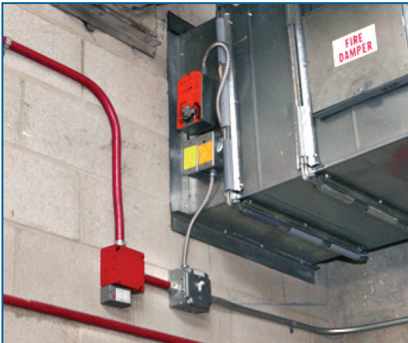
Figure 6. Fire Alarm/Smoke Control System Connection to Combination Damper (Photograph courtesy Fire Safety First)
