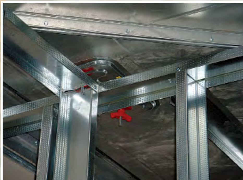
Figure 1. Blocking access doors to smoke dampers, in this case wall framing members, can make testing and maintenance disruptive and expensive. Image courtesy of David Sellers, PE, Facility Dynamic Engineer.
