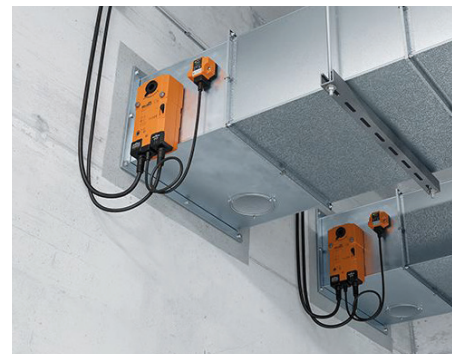
Fire damper actuators
