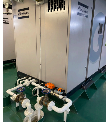
In consultation with Allseas, the 3-way system was optimised and converted to a 2-way system with Belimo Energy Valves.
