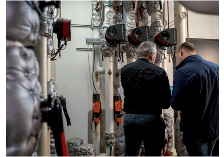
In the boiler room of the fire station: The Belimo Energy Valves
