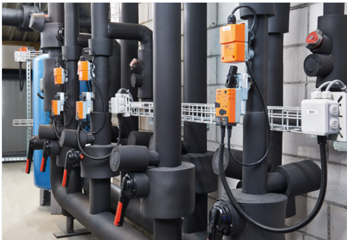
Cooling distribution with electronic pressure-independent valves (EPIV).
