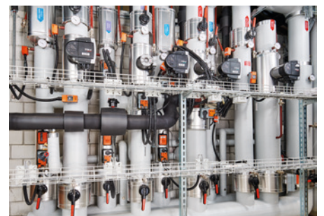
Heating distribution with electronic pressure-independent valves (EPIV), temperature sensors and temperature monitor
